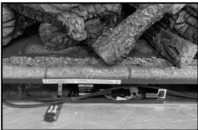
Figure 5 Location of Component Tray Underneath Firebox
