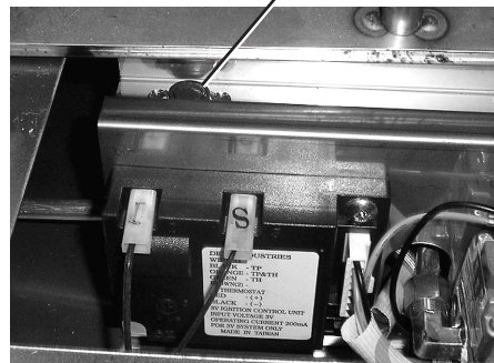
Limit Switch Location
