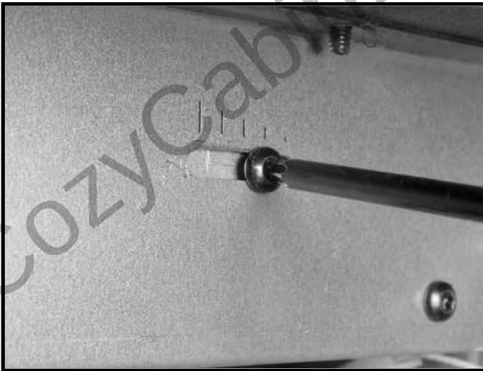
Figure 49: Initial venturi setting for natural gas.
